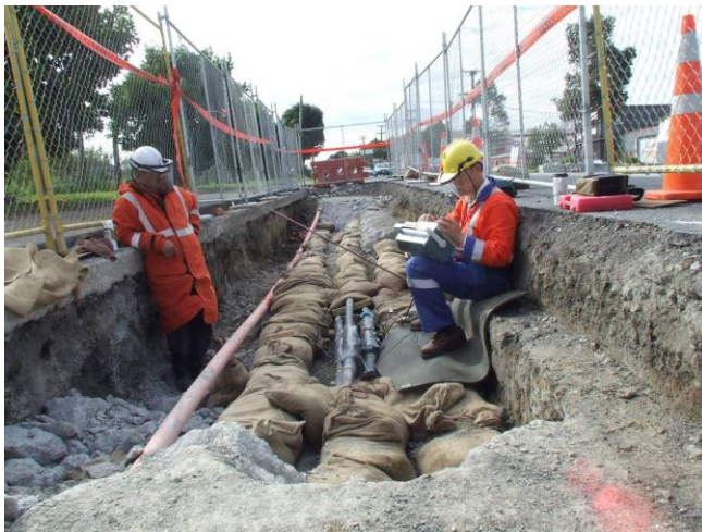
On line PD tests for the final confirmation of a PD joint to be replaced
