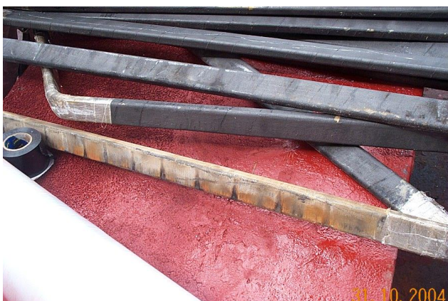
The stator bar severely eroded by PD was detected and replaced
