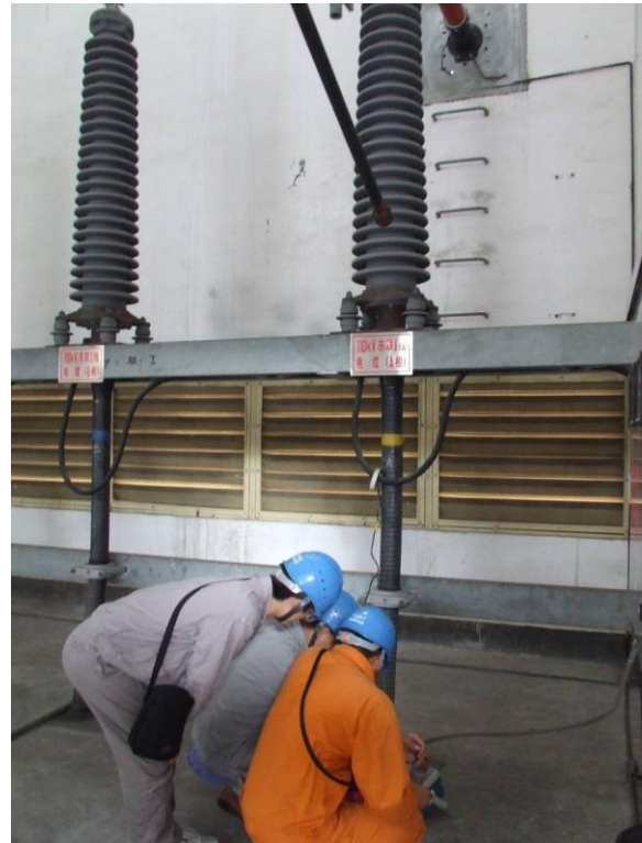
On line PD test for an 110kV cable at its termination
