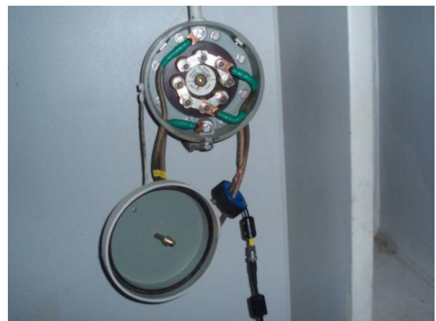
On line PD test for #5 transformer at Three Gorges plant
